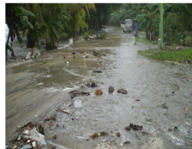
Sea water inundation event causing flooding and damage to roads
