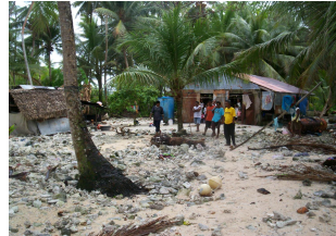
Damage from high sea surge, Lekiniach, Chuuk
